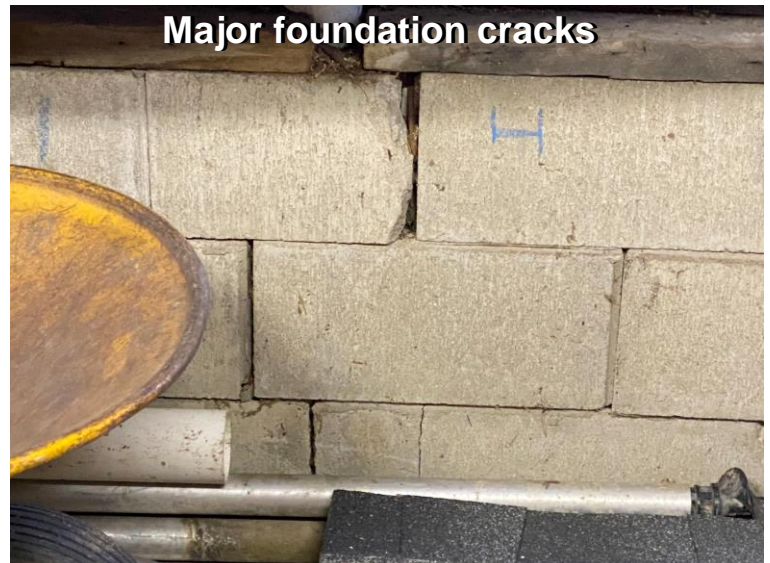
Foundation wall covered in insulation. Could be hiding damage. Damaged retaining wall is on the other side of this wall.
