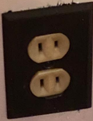
No GFCI protection
